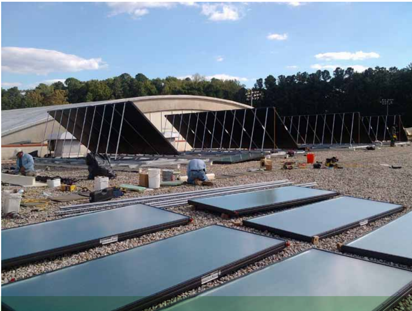
A solar thermal system was installed on the roof of Carmichael gymnasium.
